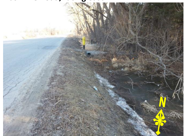
6. View of a stormwater culvert and fire hydrant located on the east side of Huntington Road at Nashville Road, facing north.
