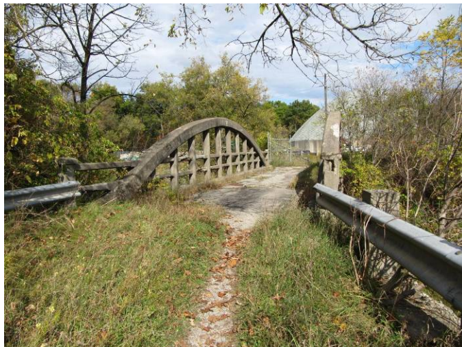
Figure 5: Former Langstaff Road Bridge in the Boyd Conservation Area, Vaughan Source: ASI, October 2010
