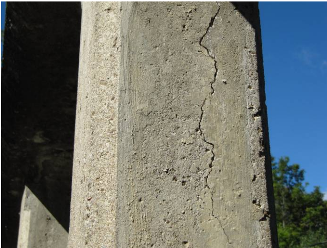
Plate 19: Detail of former patch-up work.
