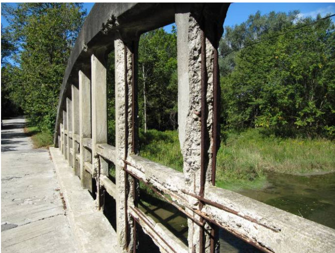
Plate 18: Detail of damaged handrail and vertical members.
