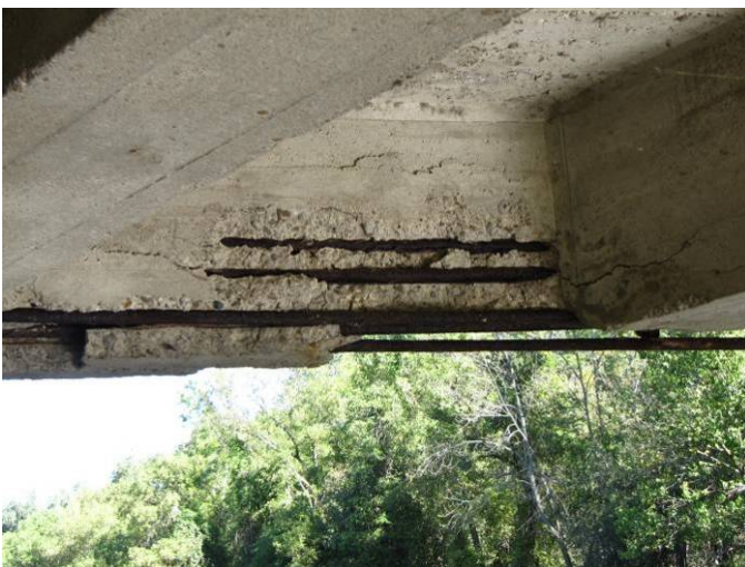
Plate 9: Detail of exposed rebar.
