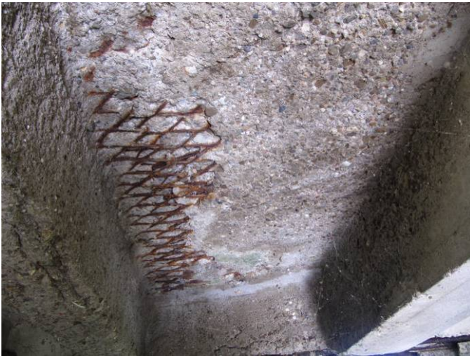
Plate 8: Detail of spalling soffit
