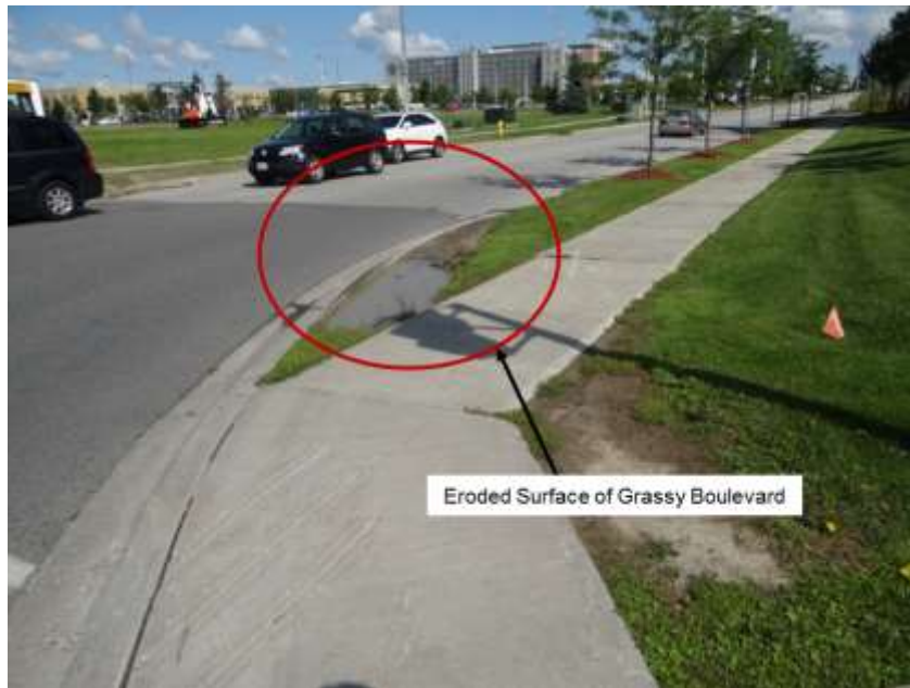
Figure 5 : Eroded Grassy Boulevard Resulting from Repeated Encroachment by Heavy Vehicles
