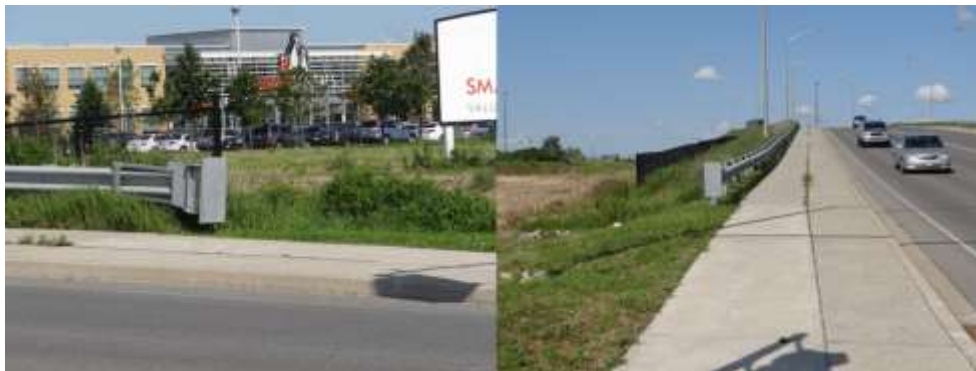
Figure 4 : Missing Object Marker Signs
