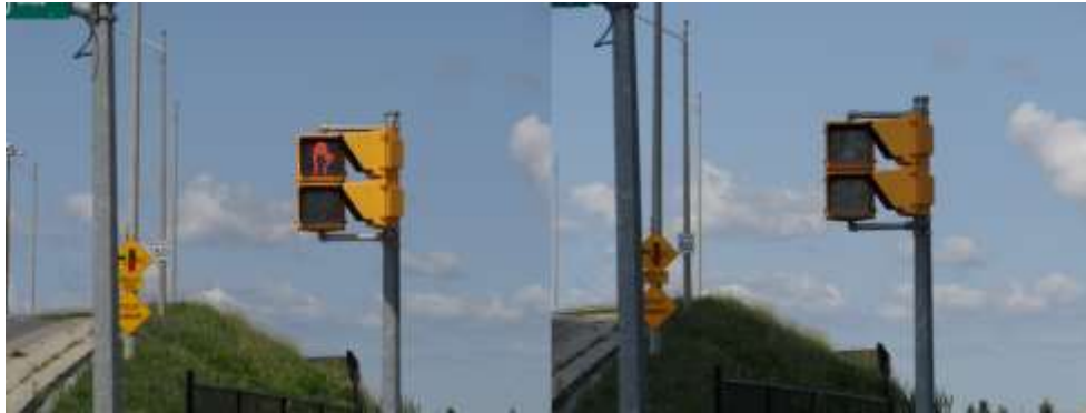
Figure 3 : Malfunctioning Pedestrian Signal Head
