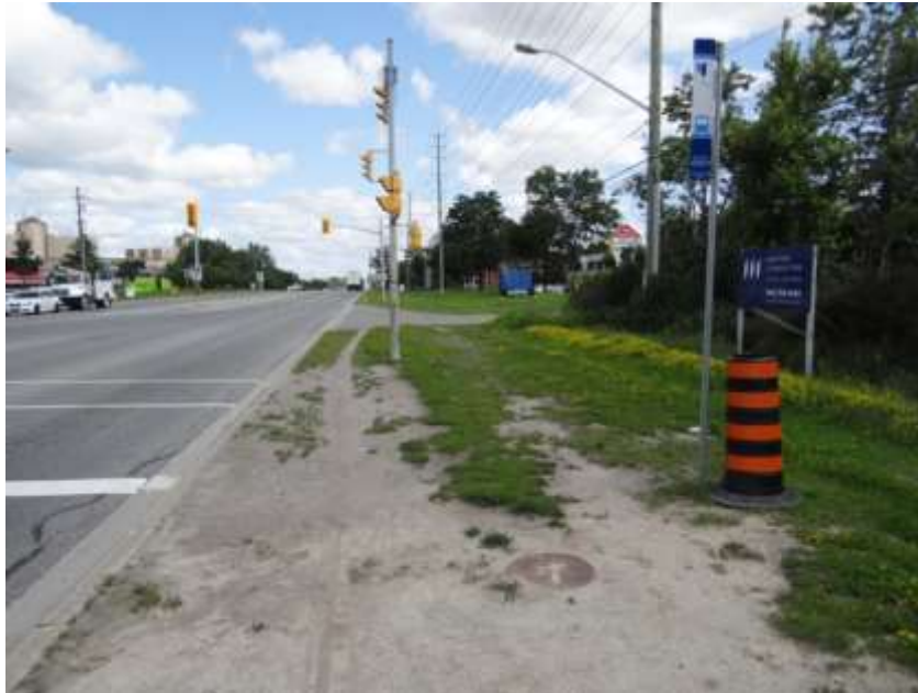
Figure 12: No Curb Ramp, Sidewalk, Concrete Pad, and Shelter at the Bus Stop (Looking North)
