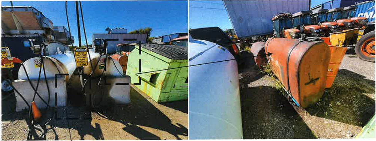
ASTs including two diesel ASTs with the associated fuel dispenser to the south of the barn and maintenance shop at 11244 Keele Street, the eastern portion of the subject site (looking west)
