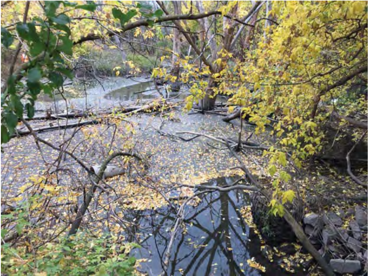
Photo 4. Back-flooded pool upstream of the failing channel stabilization works.
