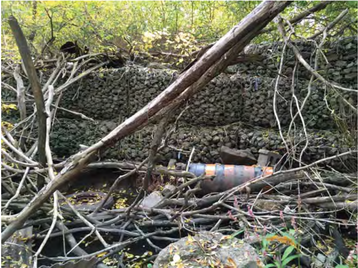
Photo 3. Failing channel stabilization works and degraded channel habitat upstream of Peelar Road.
