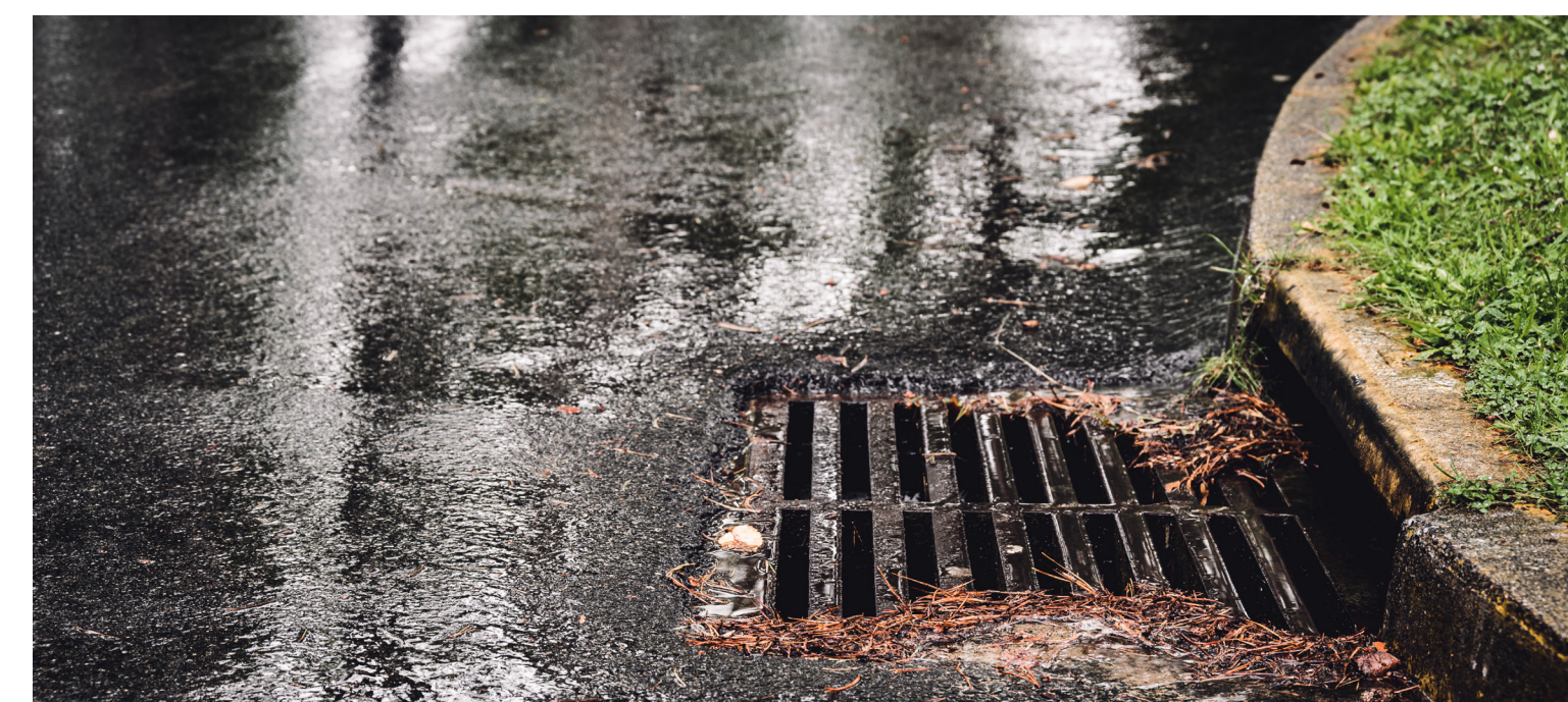
More than 22,000 catch basins
